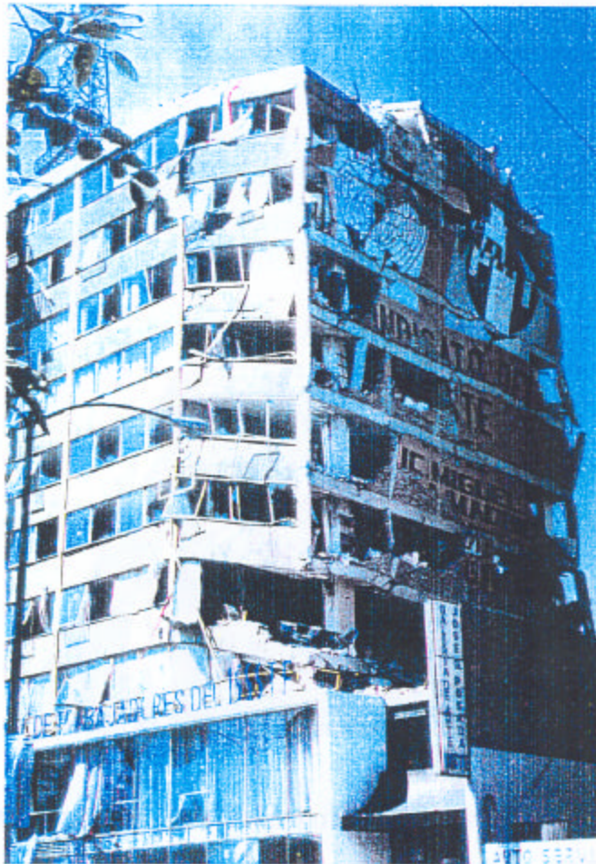
Photo 5. Failure of head-frame (corner) in upper floors because of seismic action
