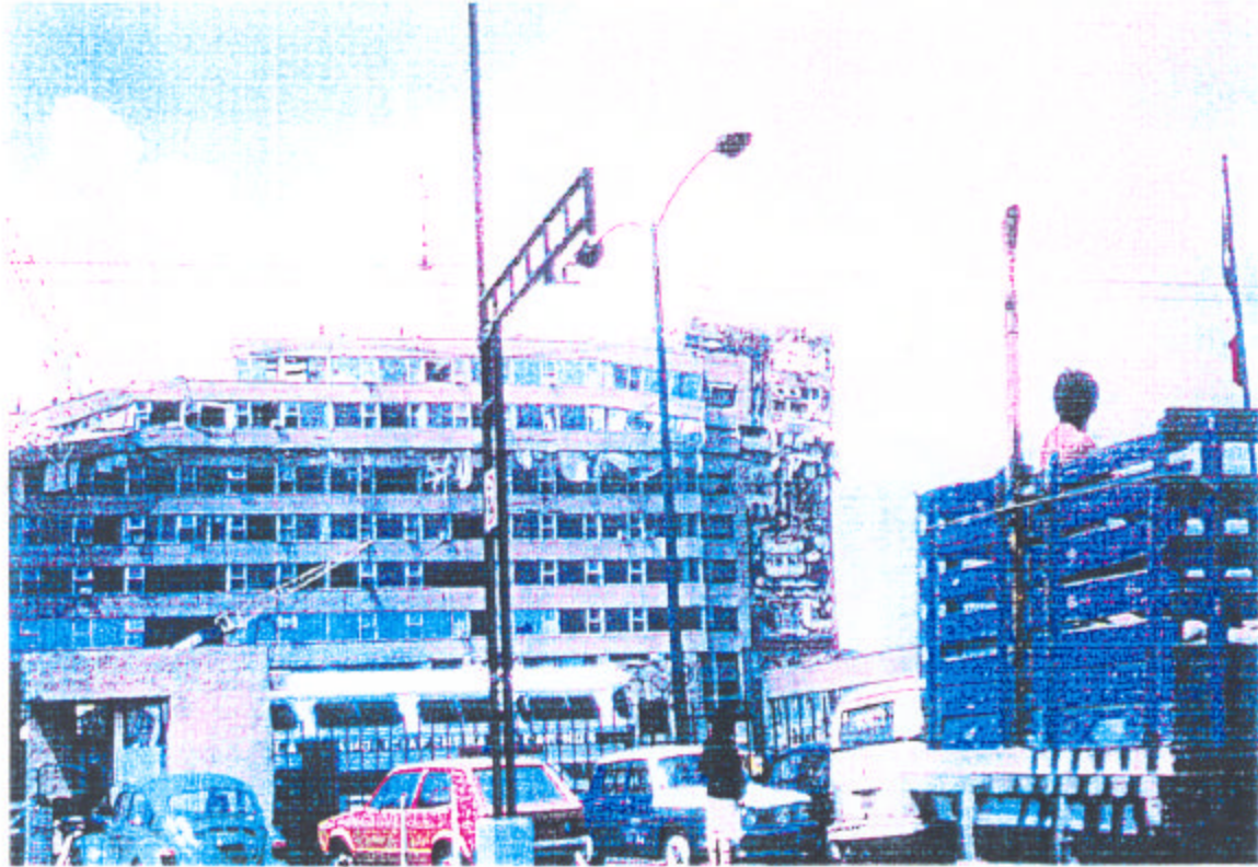
Photo 6. Failure of head-frames in the upper floors because of seismic "torsional whipping action"
