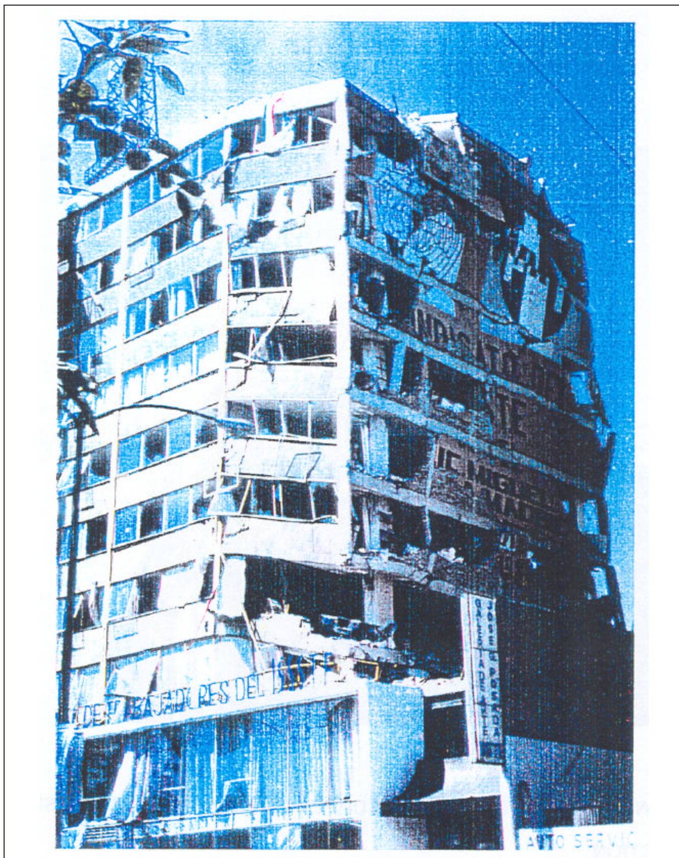
Photo 3. "Whip ping effect" in the upper floors because of seismic action
